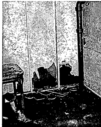
Photo 3B: Front side of wall-board looks fine, but the back side is covered with mold
